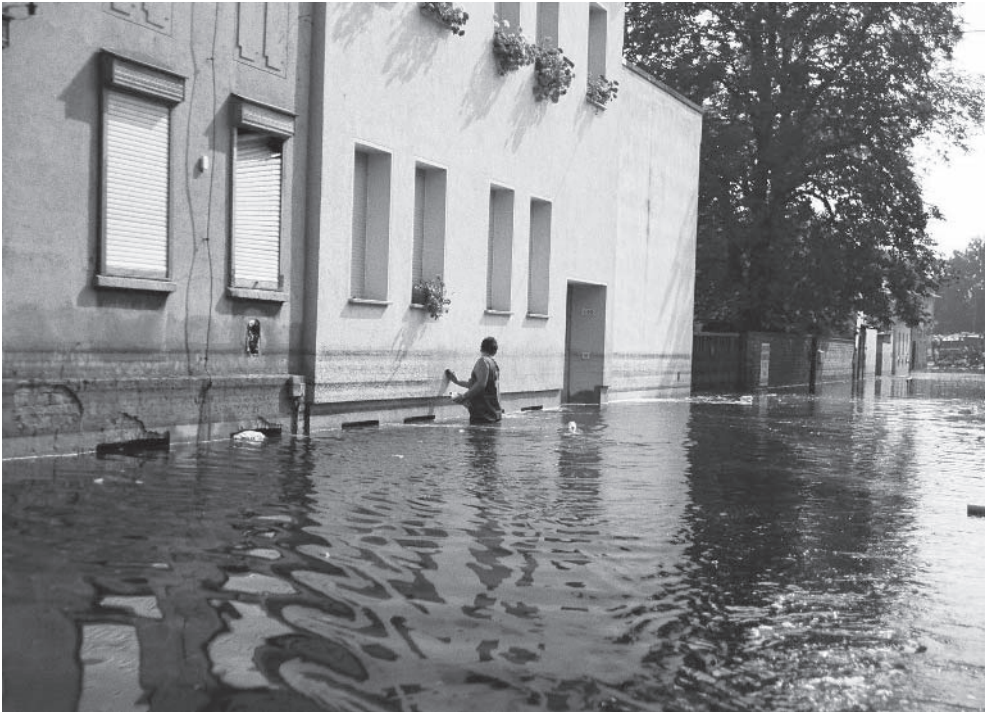
Figure 3: Resident cleaning exterior wall to remove dirt left by flood water in Waldersee near Dessau, Germany. Source: Judith Johnston, Guy Carpenter UK.
